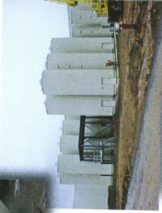
Tanks & Tank Farms
